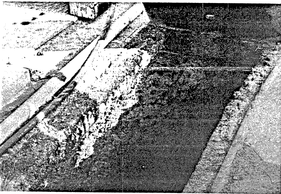
FIGURE 9. SEVERELY CORRODED CONCRETE CHANNEL IN LOS ANGELES, CA
