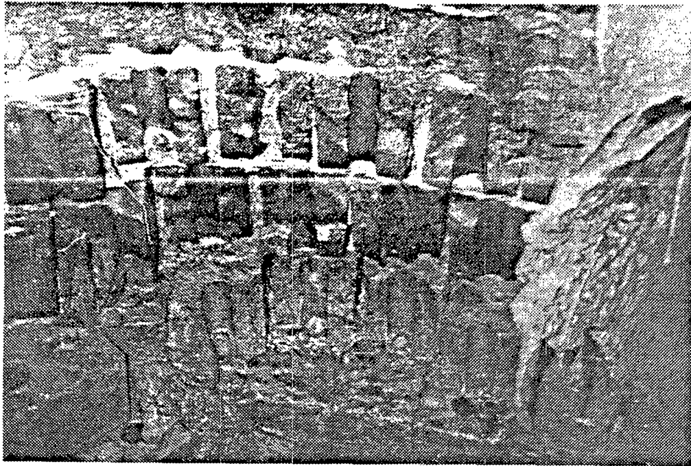
FIGURE 6. BRICK MANHOLE WITH LOOSE AND MISSING BRICKS
