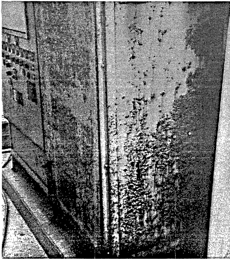
FIGURE 10. CORRODED ELECTRICAL CONTROL PANEL IN TAMPA, FL
